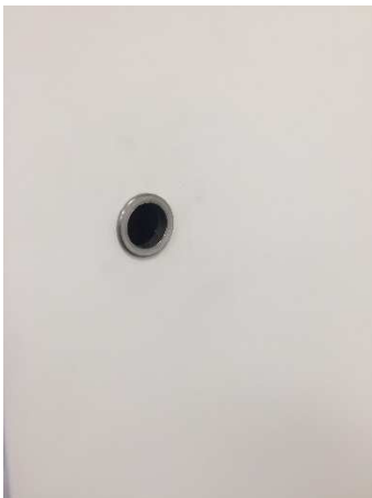
Hole within panel
